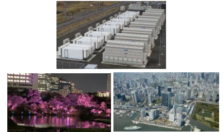
Consumption through distribution of storage batteries and power supply to public events
